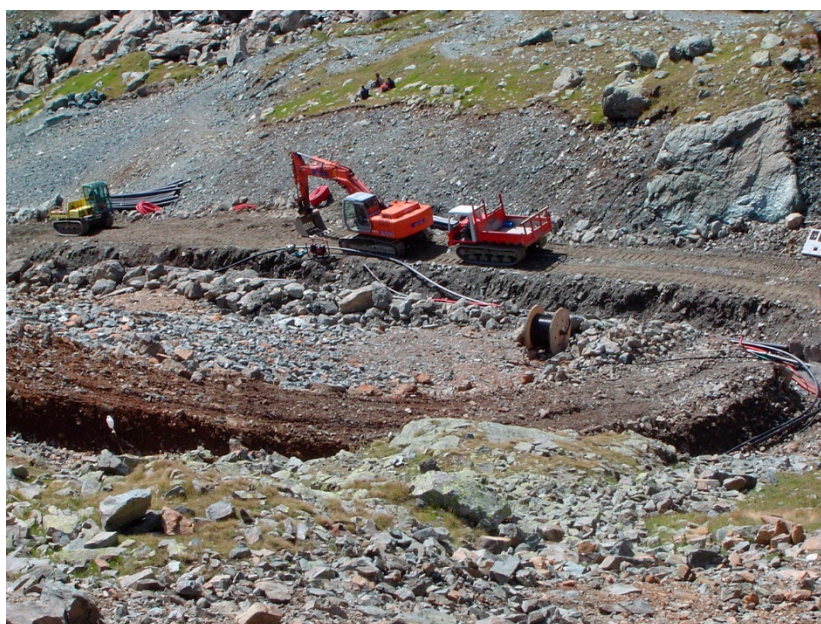
Figure 3. Construction of artificial snow-making system above the treeline in the Italian Alps (Courtesy Monterosa Ski Resort).
